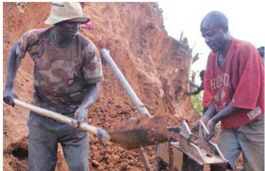
Making bricks from termite mounds located on the plots to build community storage sheds, 2015
