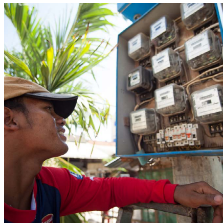
Electricity supplier monitoring the local electrical board © Germain Priour
