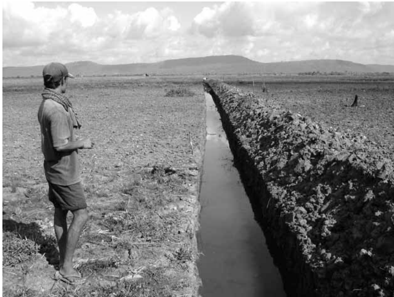
△ Bund under construction in Samrong Leu (polder 4), in May 2005. The nature of the soil made it necessary for these bunds to be voluminous, which is time consuming and reduces the useful surface of the plot. The system was only accepted if the landowners of adjacent plots shared the work and the loss of land due to the dikes equally. Refusal to participate
