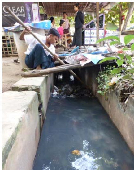
Solid waste clogging a drainage channel
